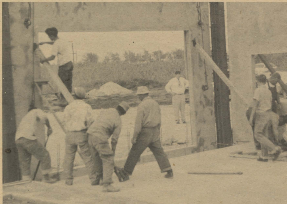
Construction rapidly progressing at new College site. Shop building already completed. Picture shows labor missionaries raising a side wall section of one of the new structures
